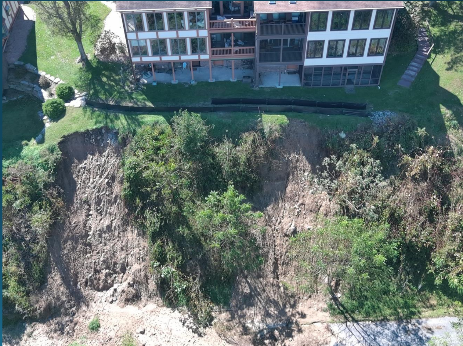
Landslides - Pinewood Circle
