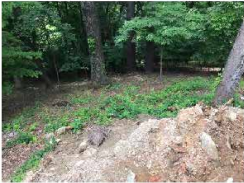
Image 9- Sedimentation on southern slope looking from driveway downhill and towards adjoining homes.
