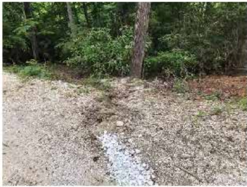
Image 21- Another stormwater conveyance channel that has developed along the driveway that is causing sedimentation in the wooded area.
