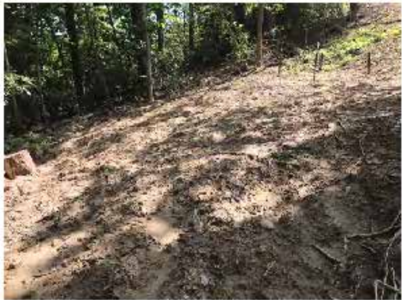
Image 15- Recently disturbed soils at new septic drainfield.
