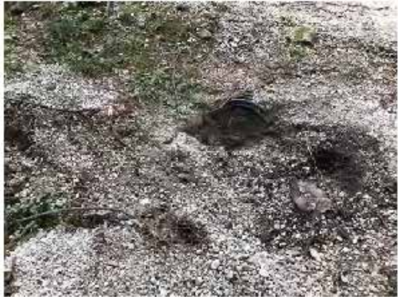
Image 27- Sedimentation from culvert #4.
