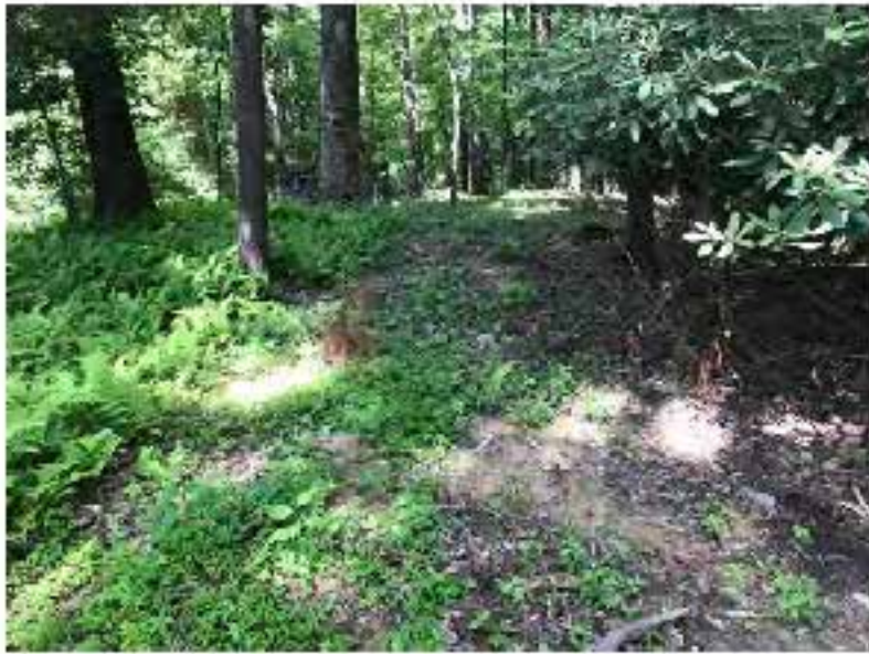
Image 16- Sedimentation down-gradient from recently constructed septic drainfield.
