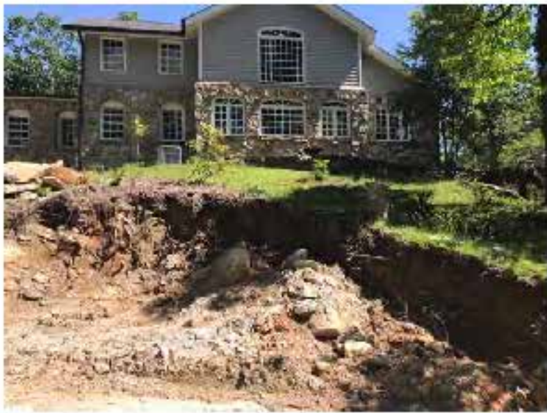
Image 5- Proposed area of disturbance on the south side of home. Proposed work here includes a hoome addition, patio, sidewalk, and retaining walls. Shows cross-section of soil profile.
