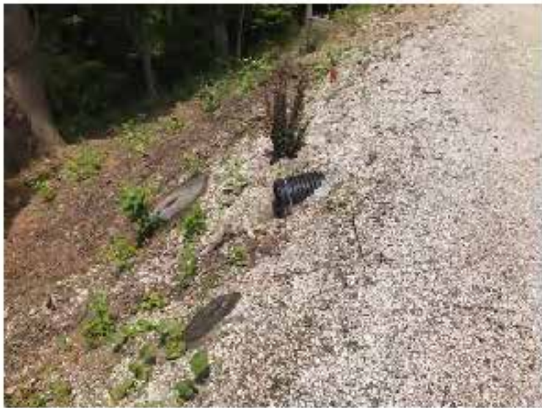
Image 22- Culvert #1 (most up-hill; near home). Erosion at outfall.
