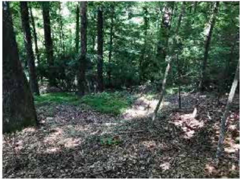
Image 8- Slump location near ravine southwest of home, and on adjoining property to the south.
