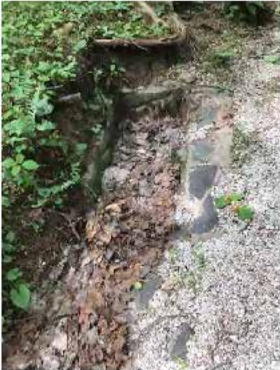
Image 26- Clogged culvert #4 (most down-hill).
