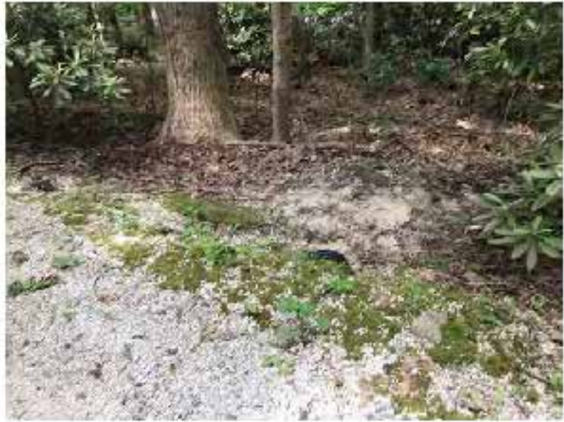
Image 25- Sedimentation from culvert #3.
